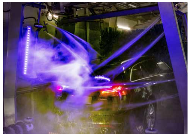
The lighting concept in the car wash tunnel highlights special performance features such as the mechanical high-pressure cleaning system.
