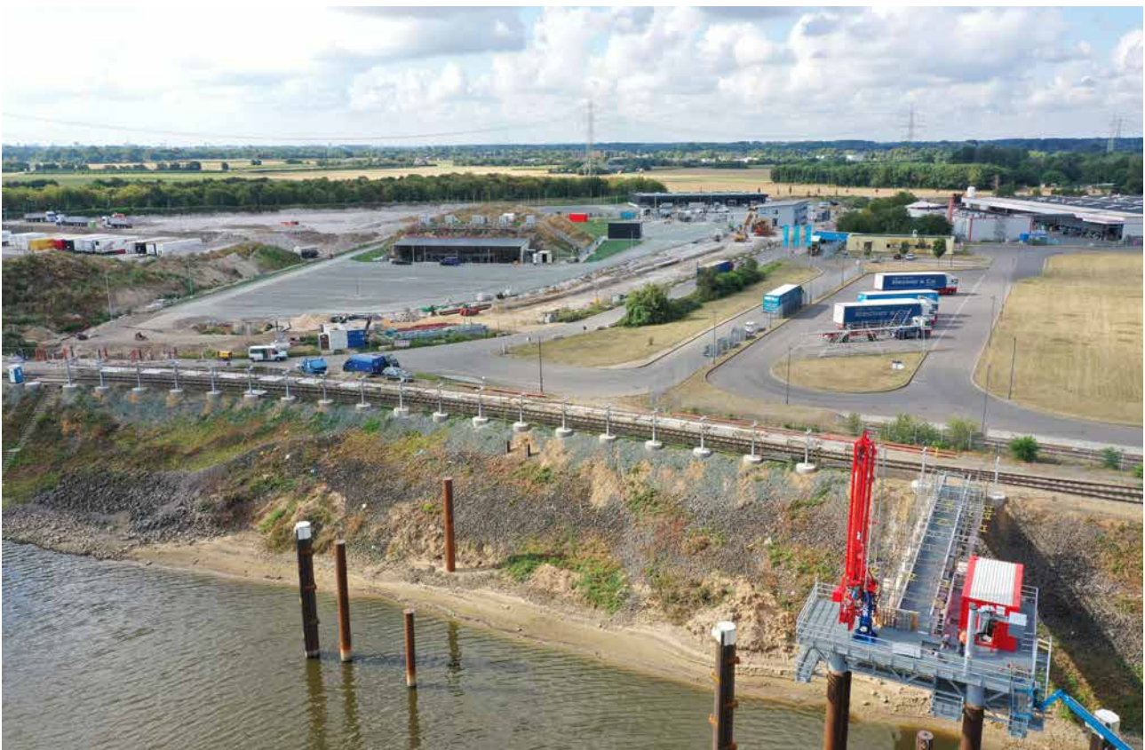
The liquid gas tank depot in the middle of building work in the summer of 2020 (clockwise from front right): Jetty, pump stand, technical equipment building, cylinder filling and office building.
