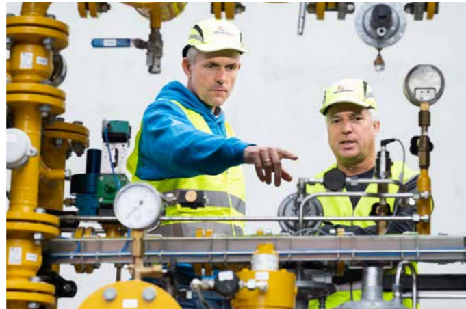
Heating transition: In a pilot project in Lochem, the Netherlands, residential buildings are being heated with hydrogen via an existing natural gas network. Alongside other partners, the Westfalen Group is also involved with its subsidiary Westfalen Gassen Nederland designing and building a plant to introduce hydrogen into the natural gas network.
