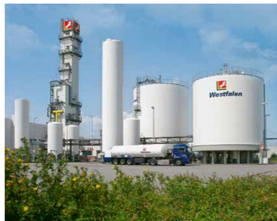
The air separation plant in Hörstel, some 50 kilometers north of Münster, was built in 1993. The Westfalen Group operates further air separation plants in Laichingen, Germany, near Ulm and in Le Creusot in France.
